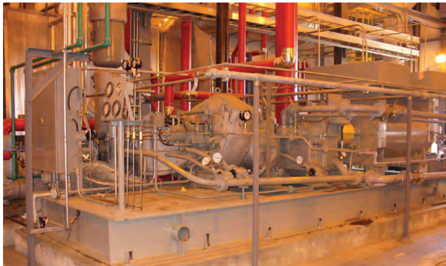
Steam let-down Turbines have been or will be installed in eight ICM-designed plants by the end of 2008.
